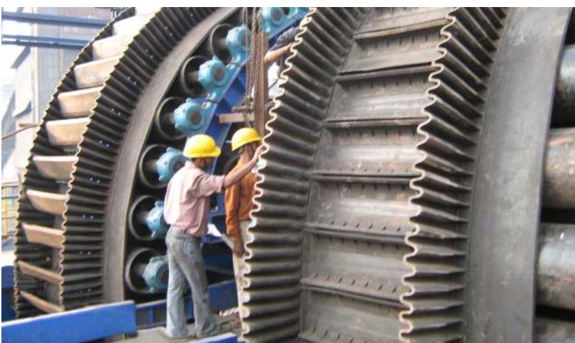
Asia's largest steep angle conveyor for handling 2X500 TPH pet coke from wagon unloading area to storage silo.
